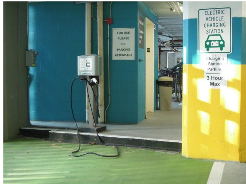
Electric Vehicle Charging Station One Broadway
