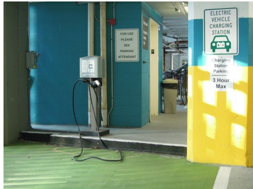
Electric Vehicle Charging Station One Broadway
